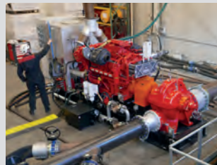
Test facilities Hydraulic testing capability up till 6.500 m 3 /hour and 40 Bar.
